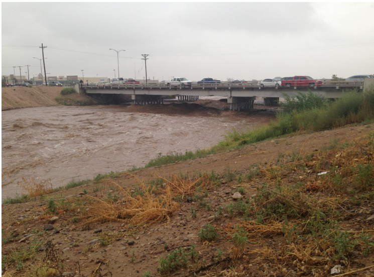
Berrendo Creek Bridge during the flooding of September 2013, Image courtesy of NMDOT.
