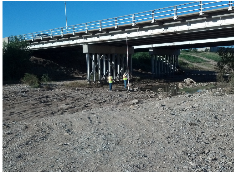
Berrendo Creek Bridge in the aftermath of the 2013 flood. Image courtesy of NMDOT.
