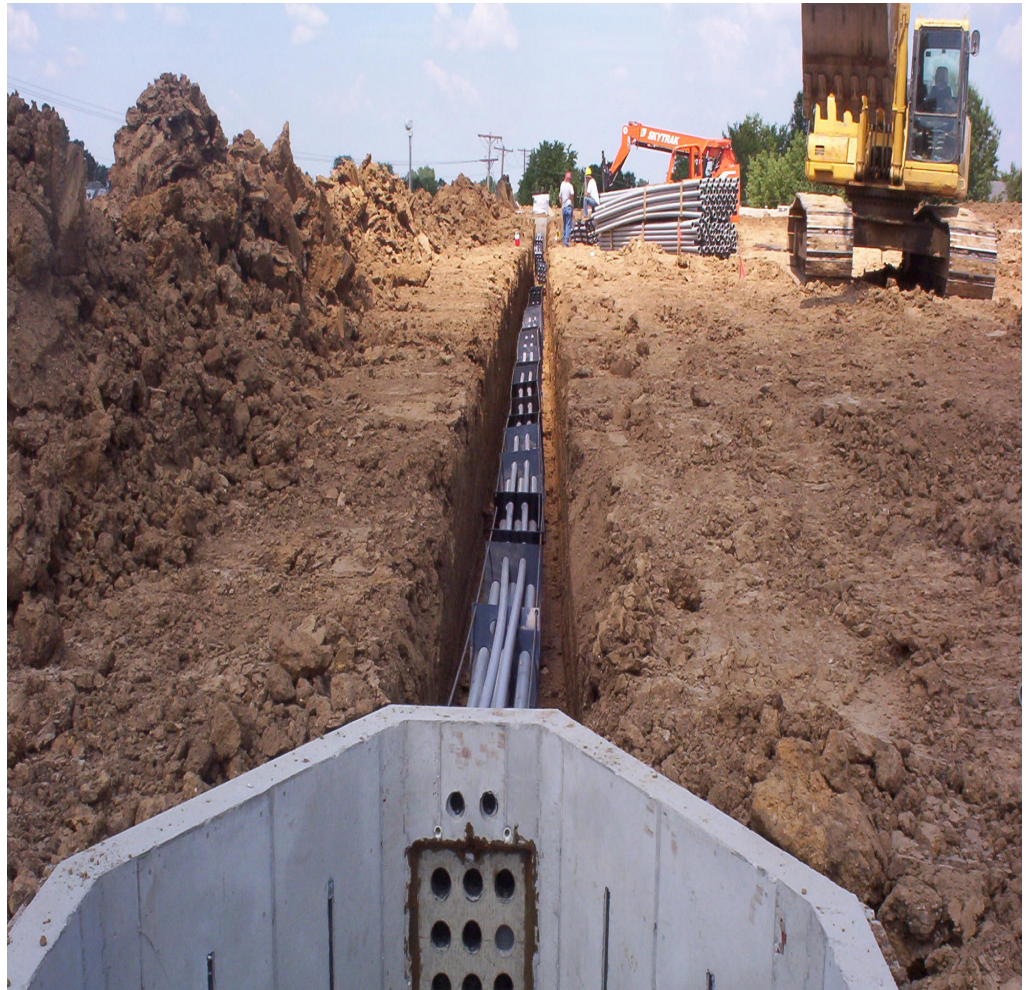
KCBPU construction of trench, conduit, and manhole structures. Image courtesy of Kansas City Board of Public Utilities
