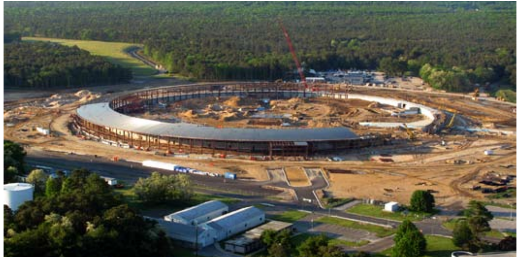
Under construction: the National Synchrotron Light Source II (NSLS-II) at Brookhaven National Laboratory.
