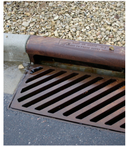
Storm sewer catch basin intake structure (Neevah casting). Image courtesy of Bolton & Menk, Inc.
