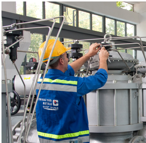
Image courtesy of GDF SUEZ Energy Romania.
