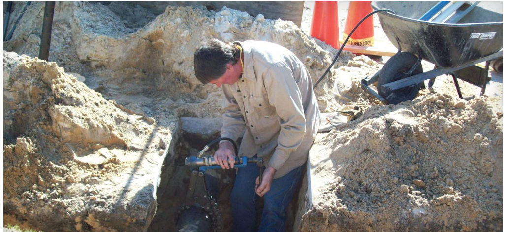
Construction teams can more easily view asset data, such as material types, necessary to complete their tasks.
