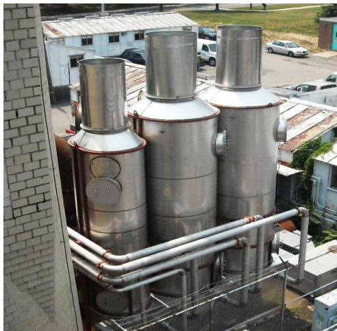
Sofame Steam Pump® in Piscataway, New Jersey. Image courtesy of Tozour Energy Services, Inc.
