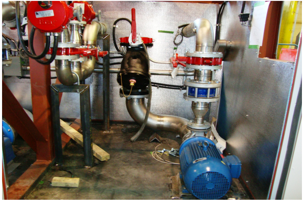
Factory-built mechanical room. Image courtesy of Sofame.
